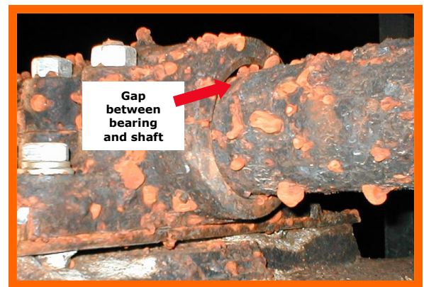
BEFORE: Shaft and bearing at Racine, WI, facility prior to replacement with AMWELL Greaseless Flocculator Bearing System.
