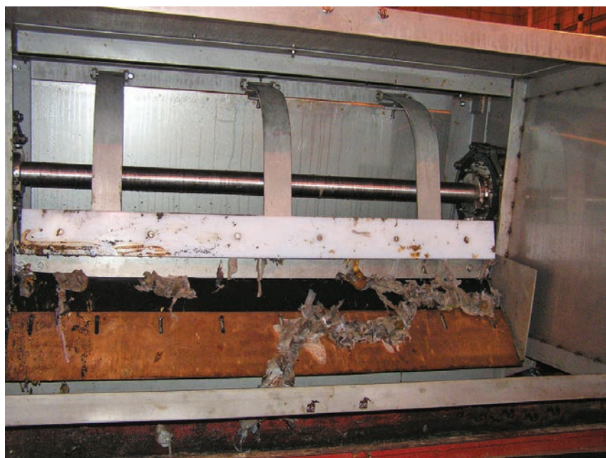
The screening system efficiently removes rags and other solid objects.
